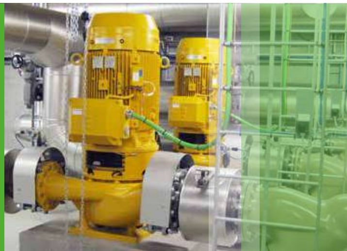
Space saving installation with vertical NSL pumps.
